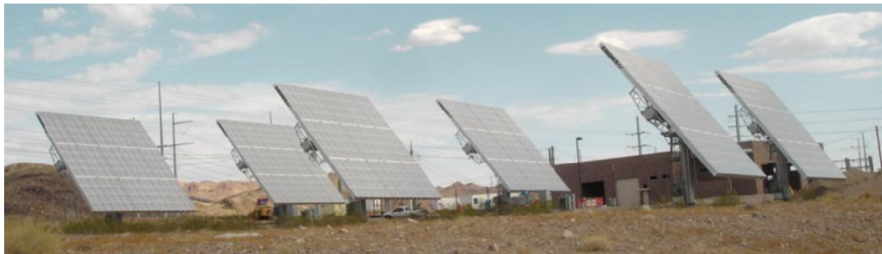
Figure 7. The 228-kW array at the Southern Nevada Water Authority's River Mountain Water Treatment Facility in Henderson, NV.
